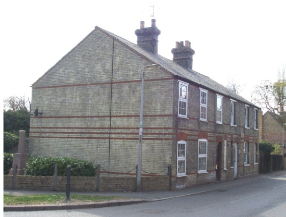
The replacement of traditional sash windows with PVCu has had a detrimental impact on the character of the Victorian terraces which front Station Road.
