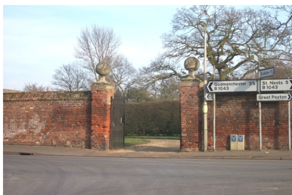
The gate piers marking the entrance to Manor House are listed . Unfortunately they are in need of some repair where damage has occurred to areas of the brickwork and the finials.
