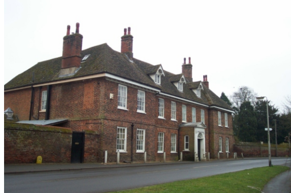
Manor House and the high red brick walls are in need of some repair.
