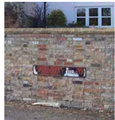
Street signage on Causeway Road which would benefit from refurbishment
