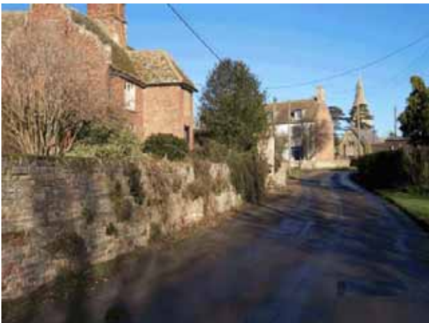
Right: an example of a boundary wall in the Broughton Conservation Area that is suffering from a lack of maintenance.
