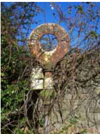
A traditional finger post that would benefit from a scheme of refurbishment
